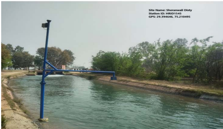
Figure 3.2: An Ultrasonic Sensor with a Boom Mount at a Canal in Haryana
