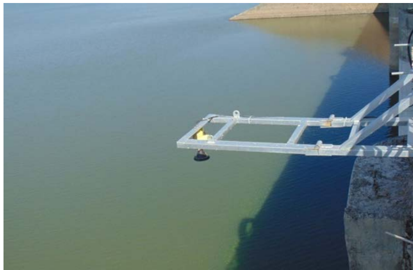
Figure 3.3: A Radar Type sensor installed on a reservoir in Gujarat
